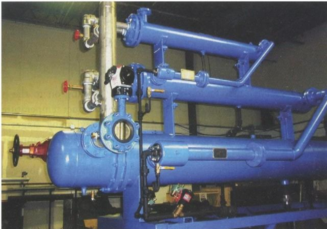
Figure 3. This three-stage Fox ejector system is the source of the vacuum cooling process
